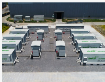
ESS Project at Haining Base
