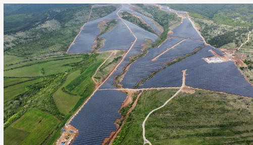
Verila Solar Power Plant in Bulgaria
