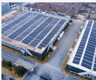
Rooftop PV System at Chuxiong Base
