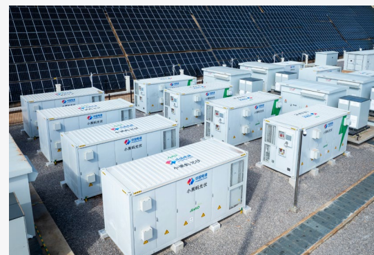
Xiaoheima "PV + ESS" Project
